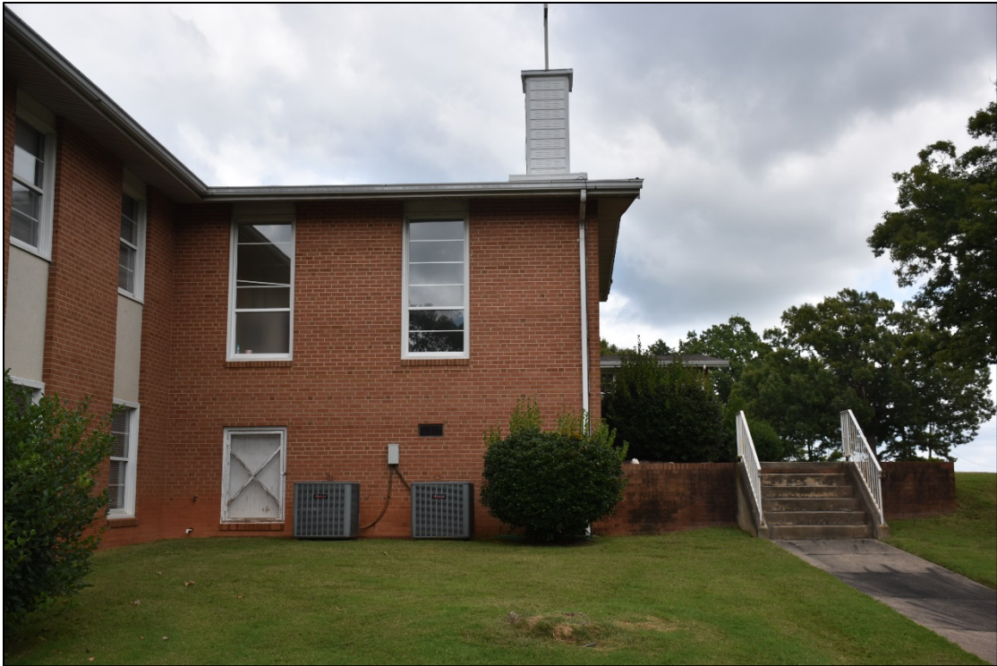
Figure 2.1.9. West elevation of western wing, West Bend United Methodist Church, facing east.
