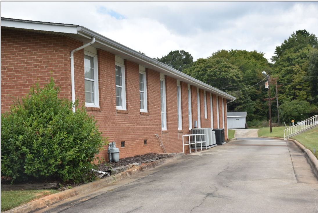
Figure 2.1.6. East elevation of eastern wing, West Bend United Methodist Church, facing northwest.
